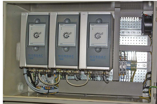
Electrical cabinet with frequency converters
